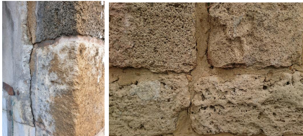
Fig.1: Pictures of the damaged historical sandstones in Tyre old city, where on the left the efflorescence case is presented, while on the right the cavities are formed due to the sub-efflorescence phenomenon, taken in January 2022.
