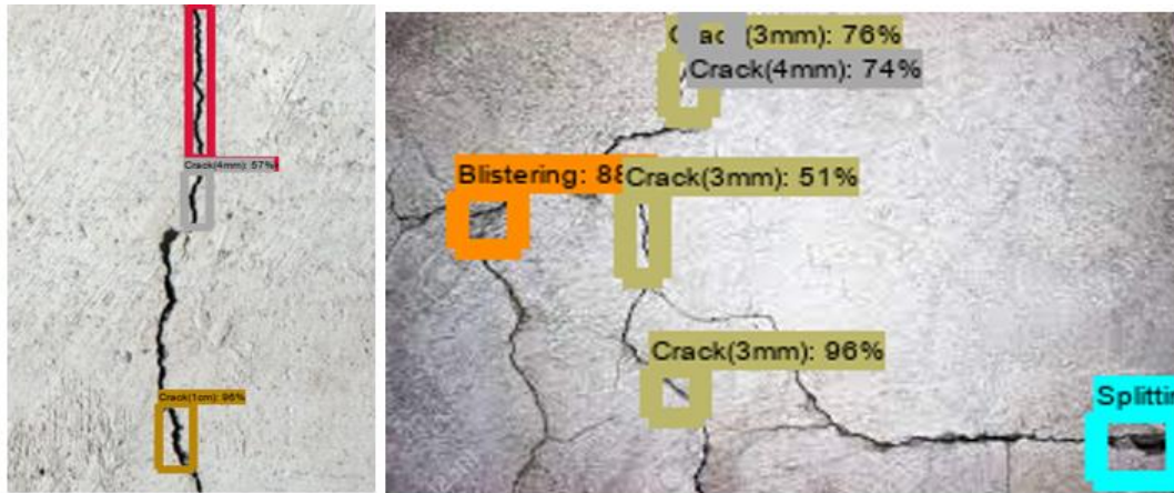
Fig.15: Output of crack, Blistering and splitting on the images (by author, 2022)
