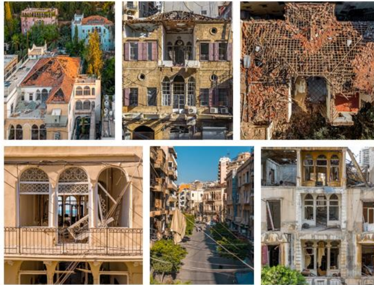
Fig.2: Footage of the mutilated heritage buildings in Mdawar, Mar Mkhayel, Achrafeyeh, Rmeil and Gemayzeh after the blast – Source: Photographed by Rami Rizk, source: Harrouk, 2020
