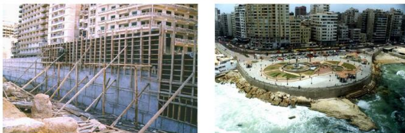
Figures 9,10: Extending the road over the sea water with reinforced seawalls; e.g. the area between (Stanley) and (Saba basha), (San Stiphano) and ( Al saraya).
