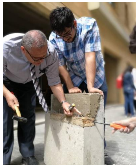
Figure 5: Concrete & wood connection problems Source: by authors.
